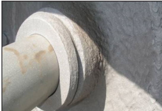
Condition of fan rotor after sandblasting
